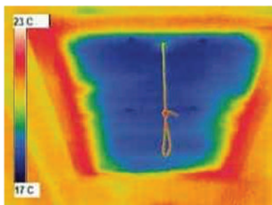
Thermal image of an uninsulated loft stairs
